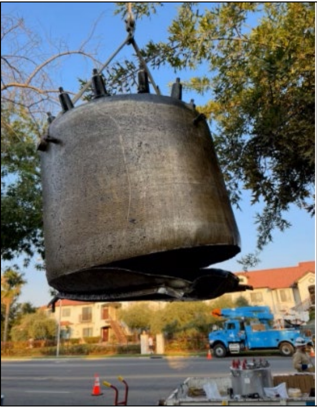
Image #2: Failed 600 Amp Trayer Switch with bottom tank weld rupture.
