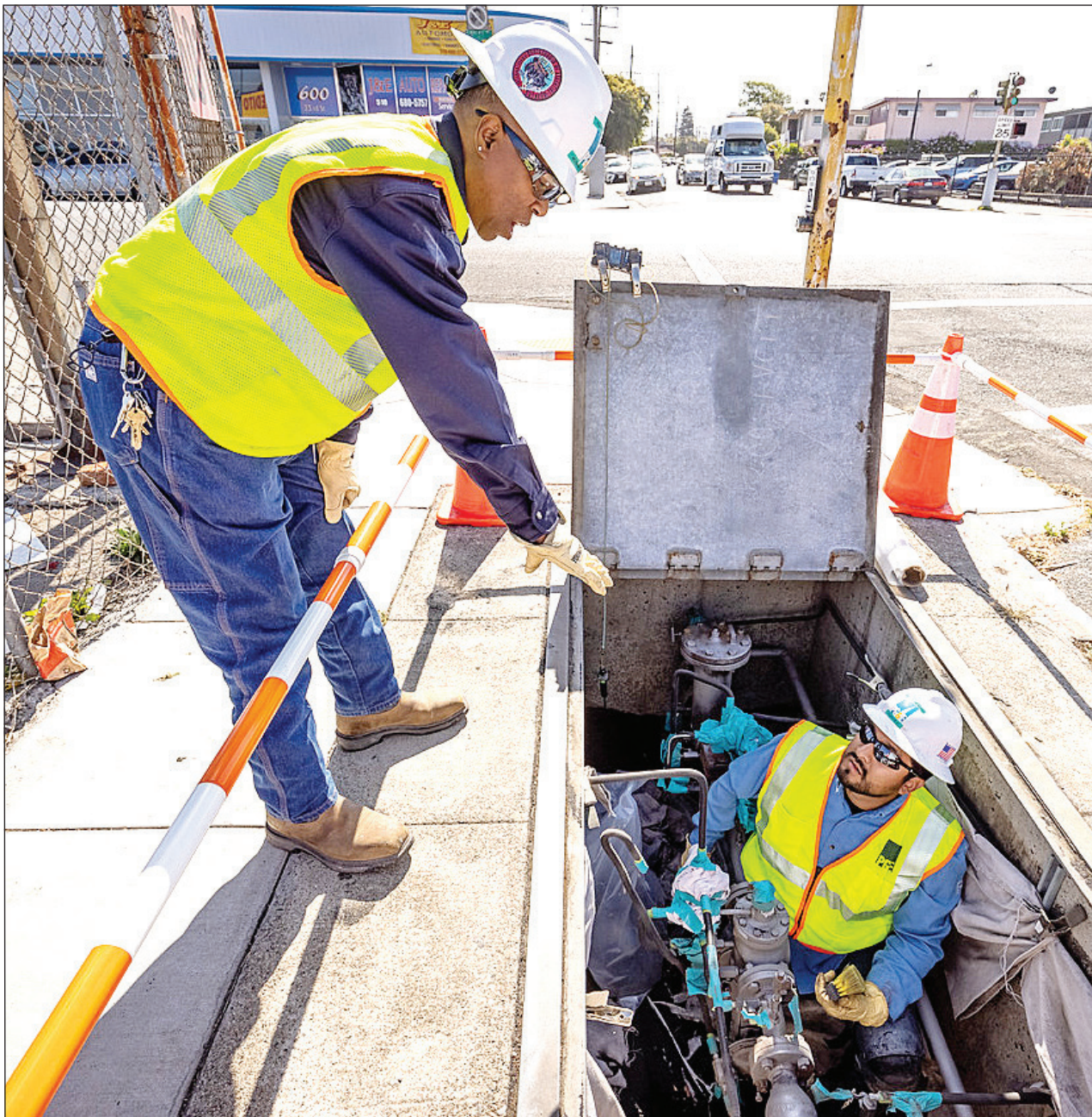
Pendleton (left) directs her crew in the vault.
