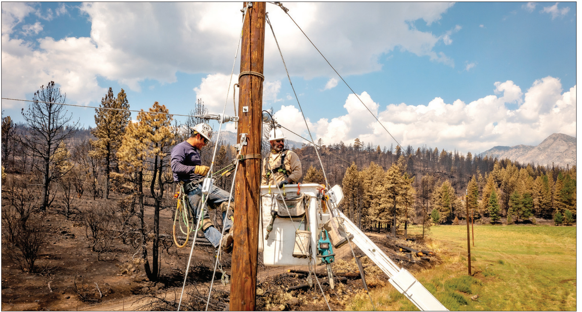
Crews from Liberty Utilities do restoration from the Tamarack Fire in Markleeville, Calif.
