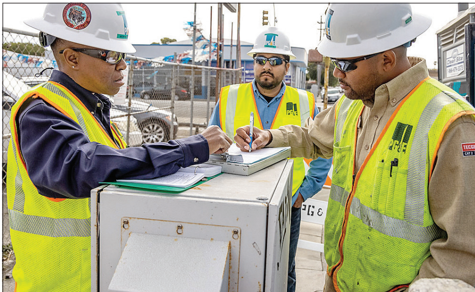
Foreman Pam Pendleton, left, with her crew, Michael Mi and Hector Olazaba, preparing to paint a gas vault in Richmond, CA.
