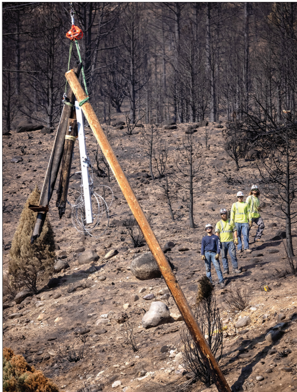
Wasatch crew Allen Birch (Foreman), Austin Peterson (apprentice), Michael Goldsby (apprentice), and Dawson Stallings (apprentice) watch as a helicopter lowers down a replacement pole.
