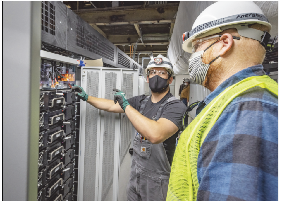
Nicholas Covello (left) and Lee Phillips check batteries.
