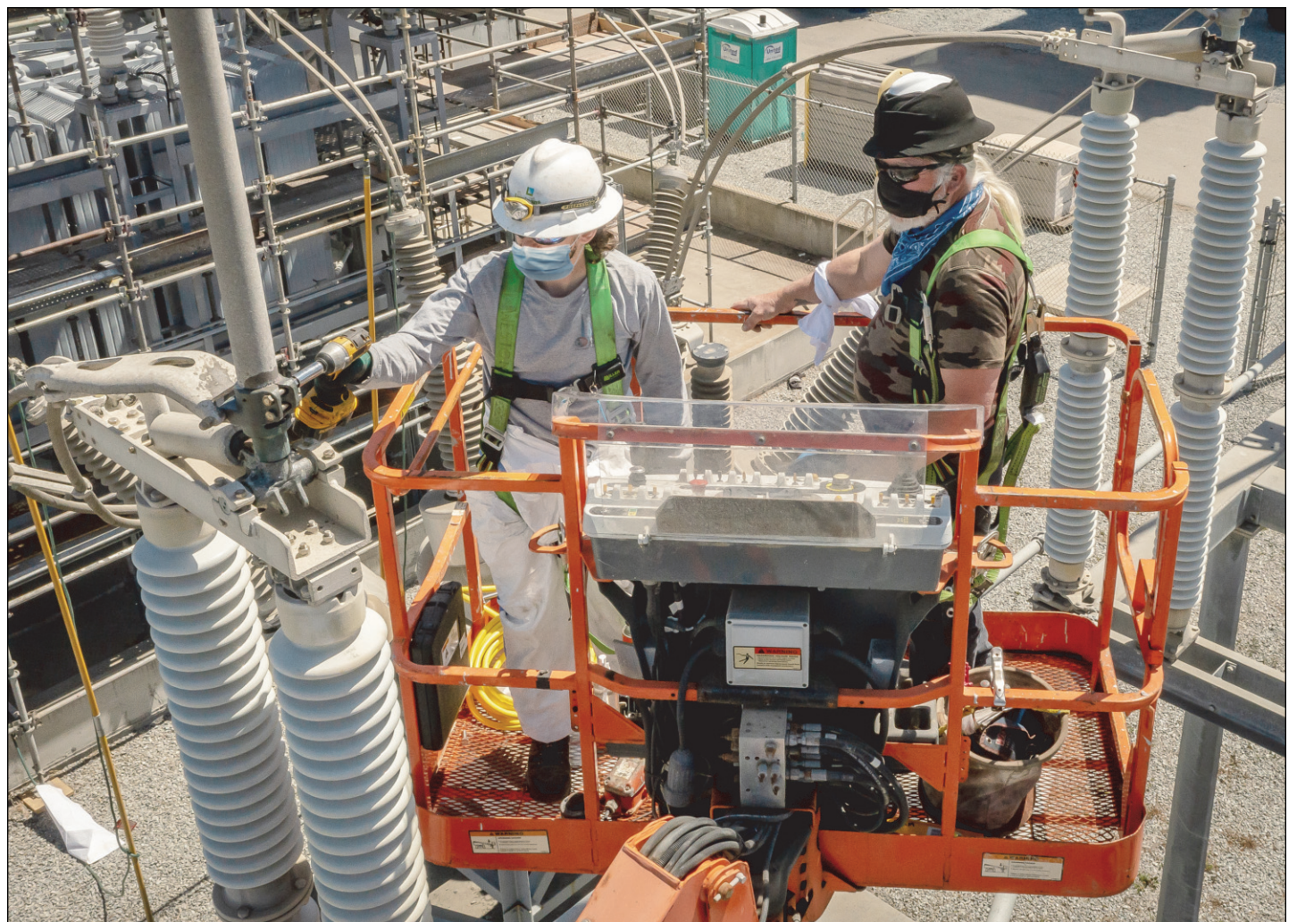
Power Plant Techs Doug Bailey (Camo) and Weston Miller (left) do maintenance.
