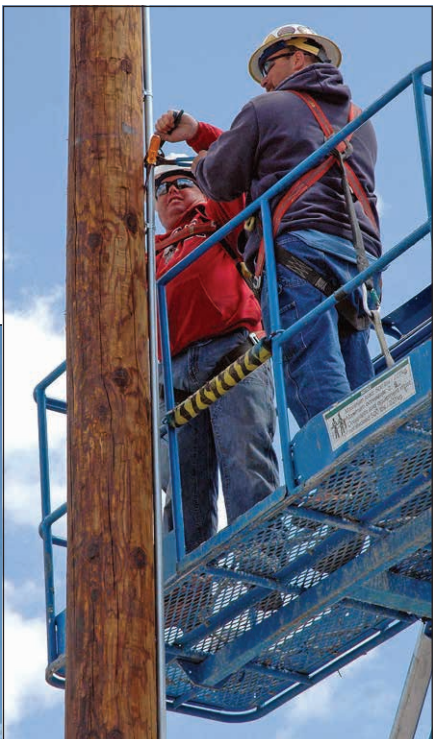
Kevin Bellows (left in insert) and Ben Shelton install light box for yard light.
