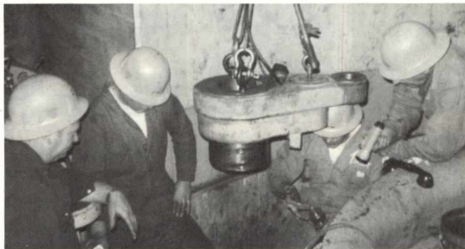
Shown above from left to right are: Mark Burns, Jr., Electrical Machinist; Dude McMaster, Appr. Elec. Mach. and Helpers Jim Tiner and Ray Heath installing wicket bell crank.
