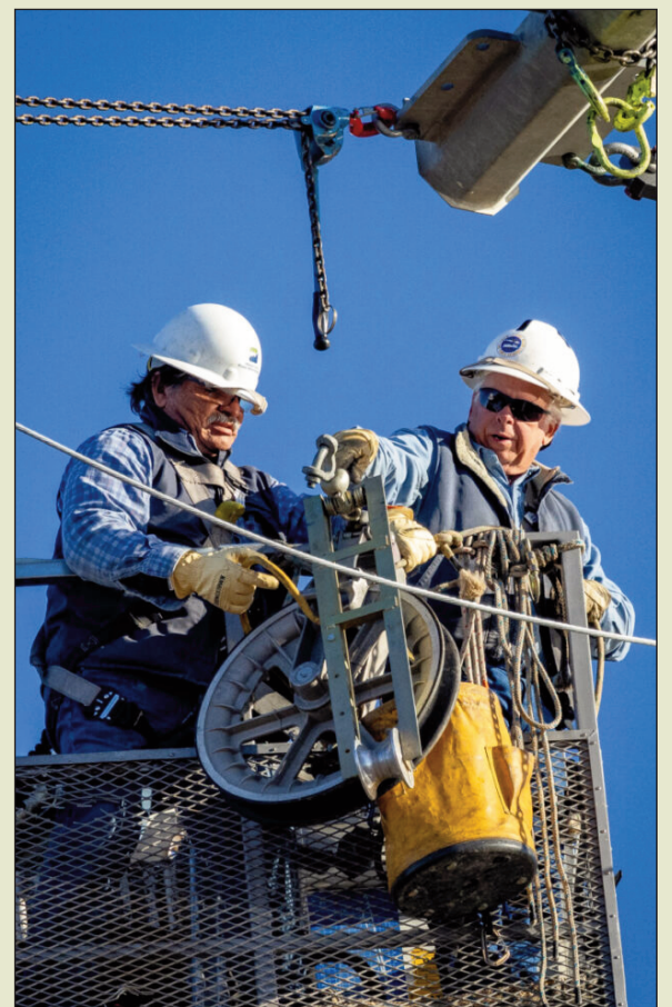
Journeyman Linemen Joel Carillo and Dave Horton from WAPA sag fiber on a new transmission line to Beale Air Force Base in Marysville, Calif. on November 12, 2024.
