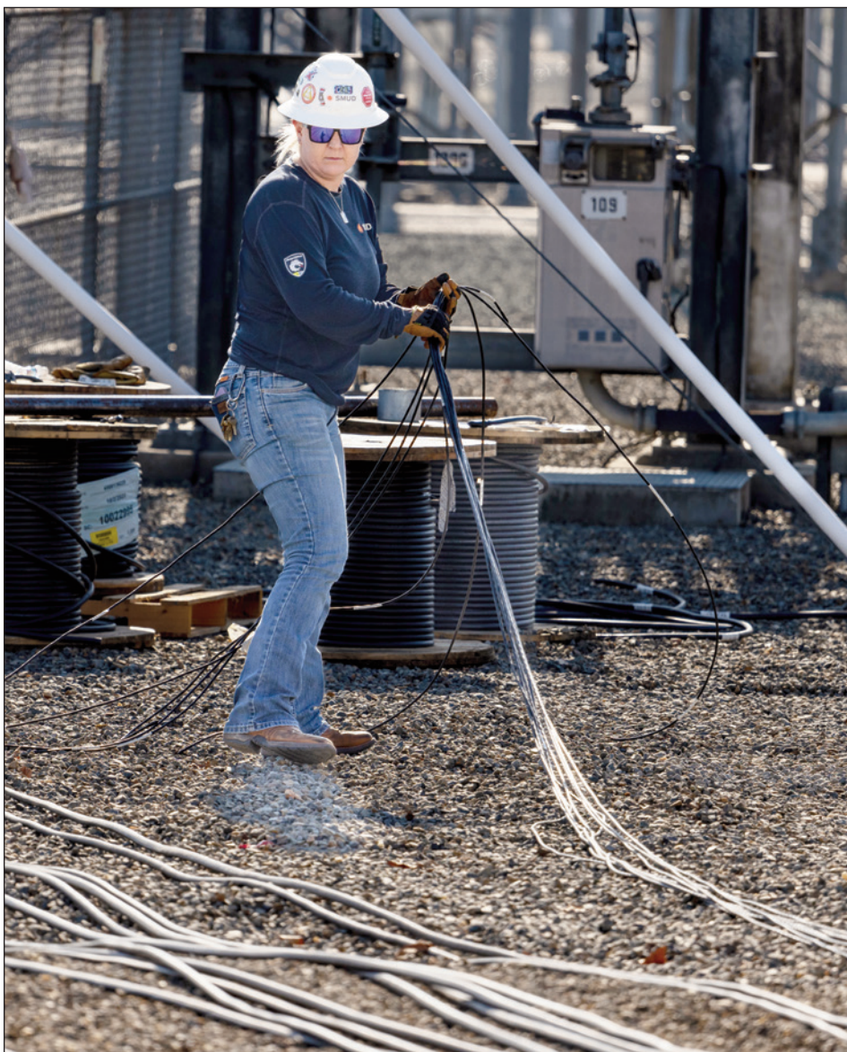
High Voltage Substation Electrician Karyn Newmark works at the Hurley Substation in Sacramento.
