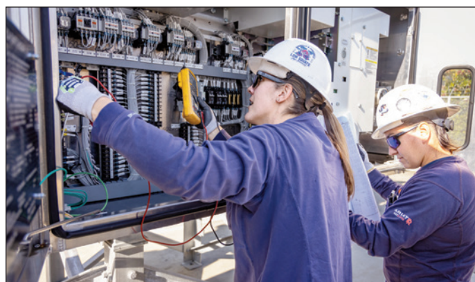
Apprentice High Voltage Electrician Yesenia Vega and Apprentice High Voltage Electrician Megan Kilgore work at the Hurley Substation in Sacramento.
