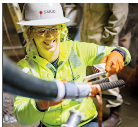
Foreman Cable Splicer Heather Andersen splices a cable in an electrical vault at the Sacramento Convention Center.
