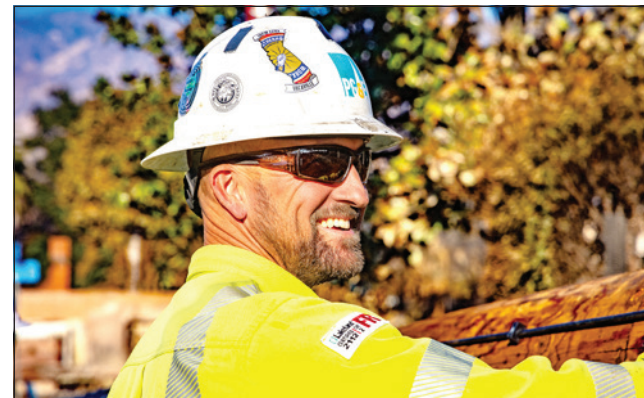
Apprentice Lineman James Negranti with the PG&E Los Padres GC crew is repairing damage from the Eaton fire and rebuilding an entire circuit, cutting it over from 4KV to 16KV.
