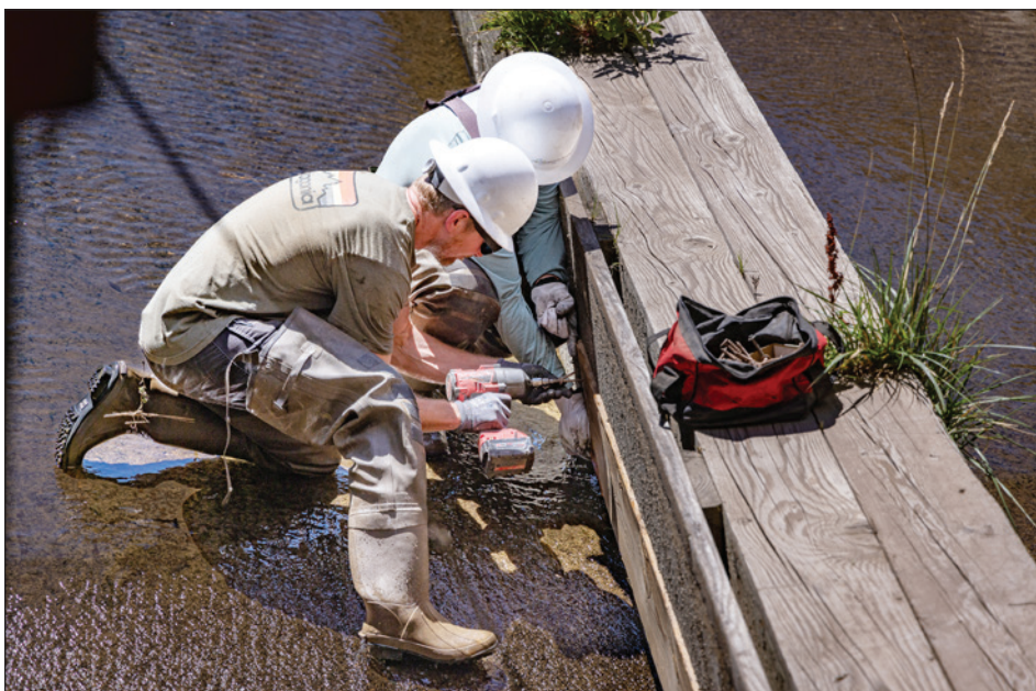
IBEW Local 1245 members from Truckee Meadows Water District fix the water canal debris diverter at the Verdi Hydroelectric Plant.
