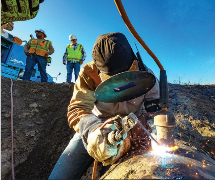
PG&E GC Gas Crew weld a valve onto a 22” line in Livermore, Calif.
