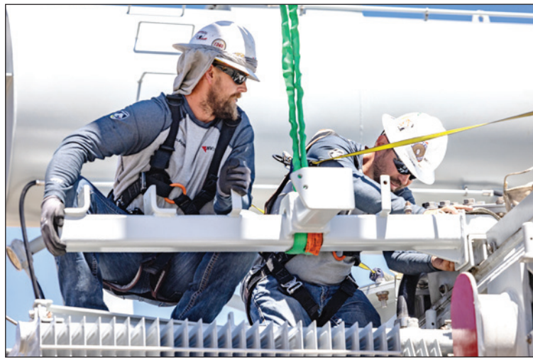
IBEW Local 1245 members from NV Energy assemble a new transformer at the Northwest Substation in Reno, Nevada on August 14, 2024.
