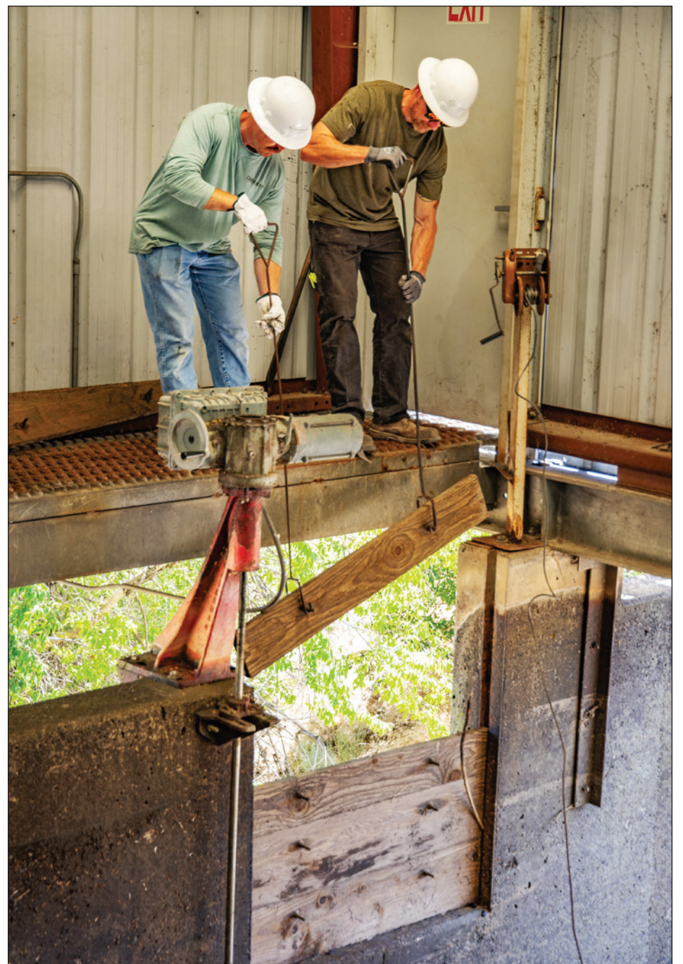
IBEW Local 1245 members from Truckee Meadows Water District replace boards to divert water to the turbine.
