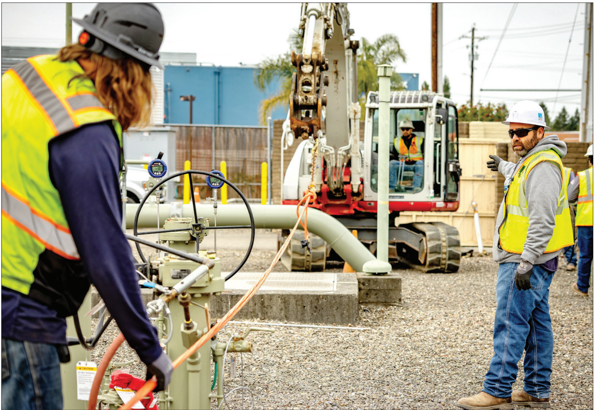
IBEW 1245 members from PG&E prepare to perform an inline inspection on a gas main at the Santa Rosa compressor station.
