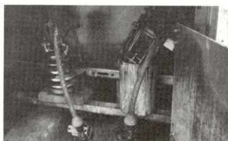
Shown above is the damaged Kyle Switch.
