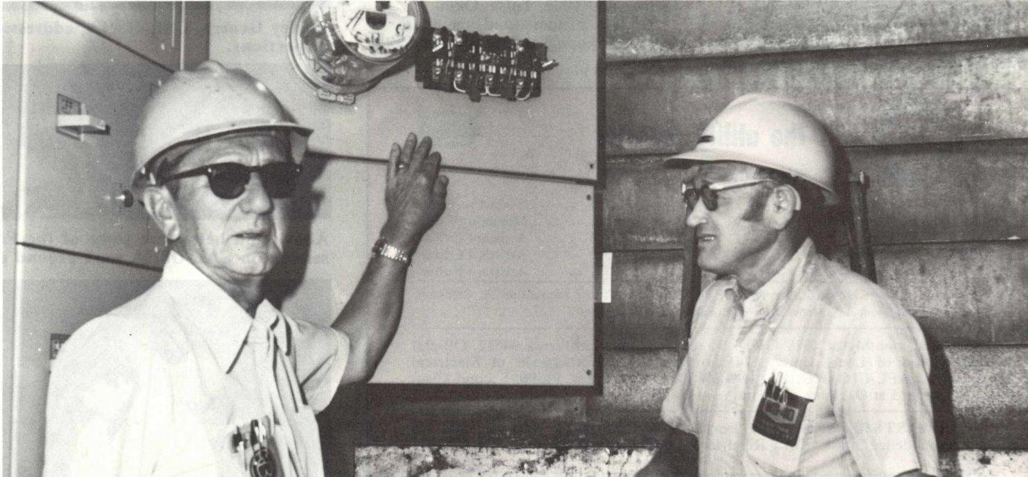
Shown here at a new meter box are: (L to R) Aaron Bayer, Meterman and Bob Linton, Electrician.
