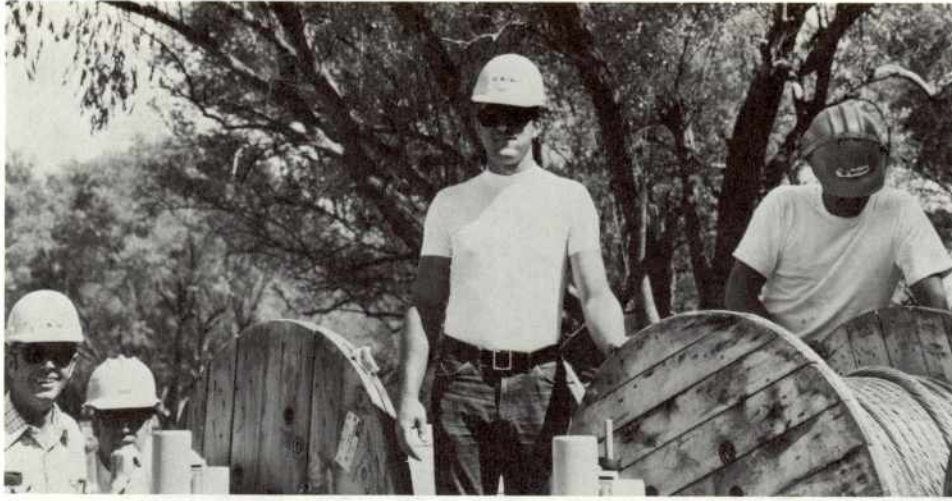
This photo shows underground crew at work. Shown in this photo are: Jim Burke, Foreman, Corky Coons, Lineman, Don Powell, Lineman, and Rod Goehring, Apprentice.
