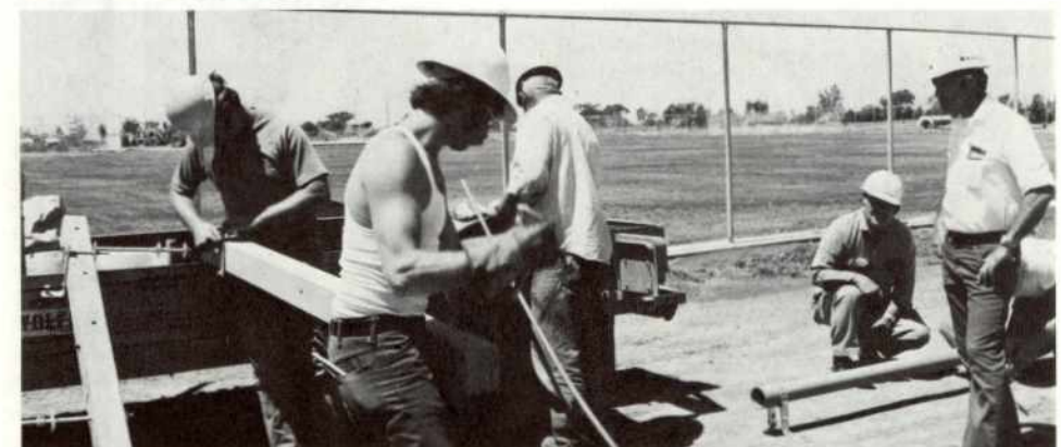
An underground crew is shown working in a park in Elk Grove, Calif. Members of the crew are Al Glidden, Sarge Wilkens, Glen Campbell, Jim Phelan, Lynn Wallace and foreman Lou Earles.
