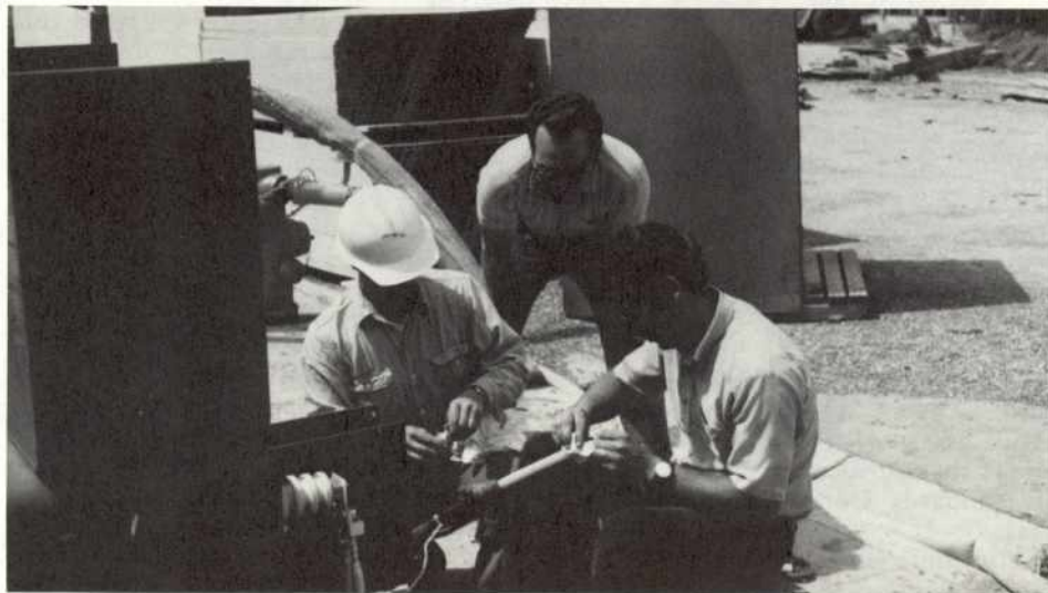
Shown above are members working on transformers: from left to right Joe Don McMasters, Lineman; John F. Hartley, Electrician and Larry Giovannoni, Appr. Lineman.
