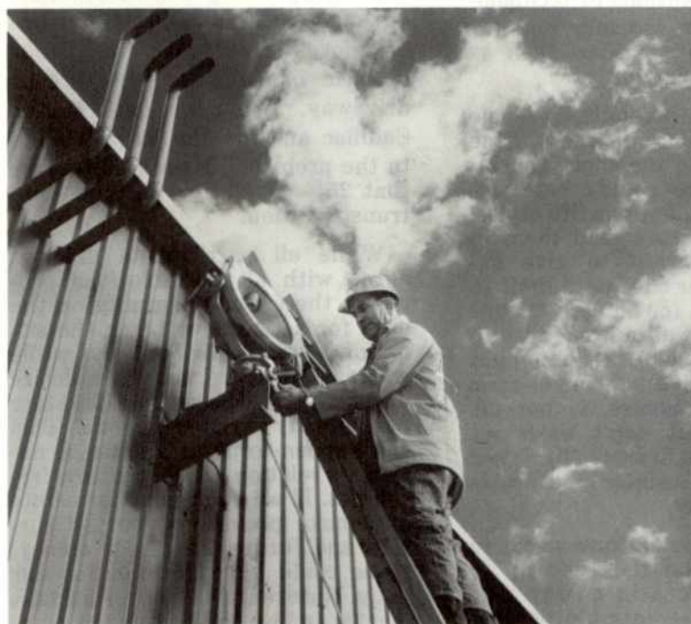
Shop Steward Jim Smith, Sr. Mech., is shown changing a light fixture at Station #10 (Kent), approximately 100 miles southeast of Portland, Oregon.
