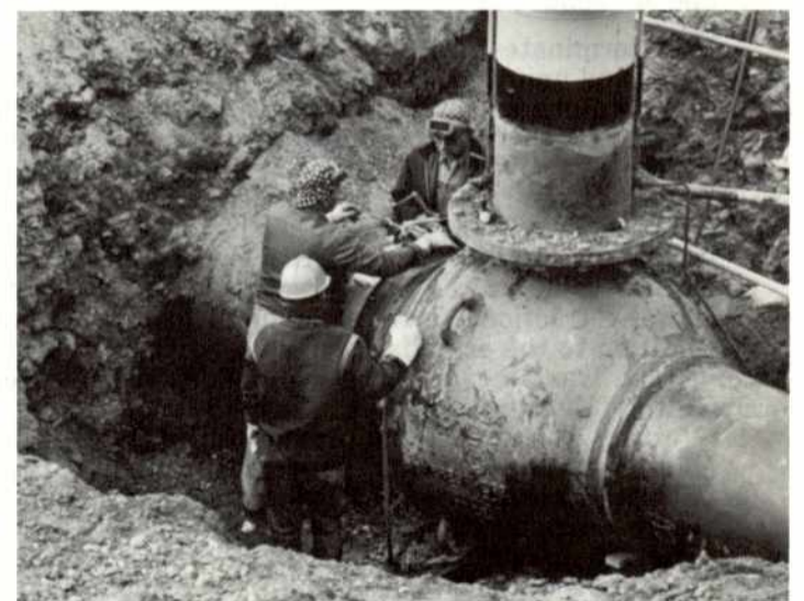
Clockwise, from front, Jim Yount, Dick Perry, Myron Power and Deaver Noland are shown removing the station suction valve at Station #6, Rosalia, Washington.
