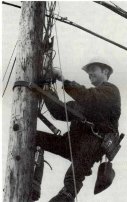
Installer repairman Jerry Will is shown as he connects a phone service at the pole.
