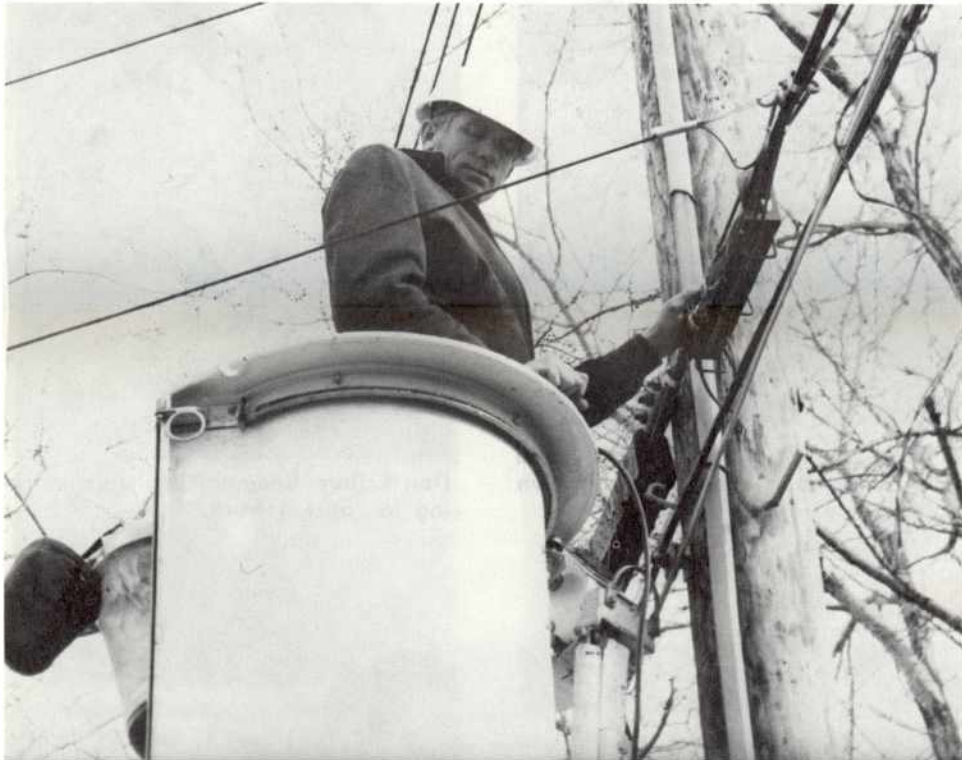
Les Hatch, Cable Splicer, is shown in a "bucket truck" as he works on a splice.
