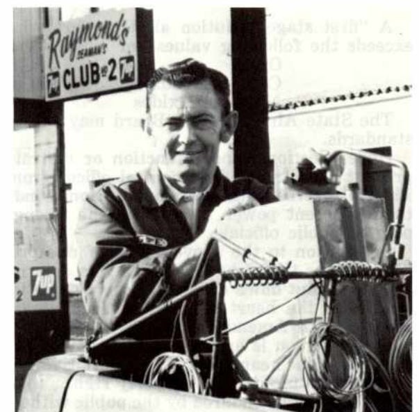
Herb Dutra, Gas Service Mechanic, is shown preparing to install a new meter.
