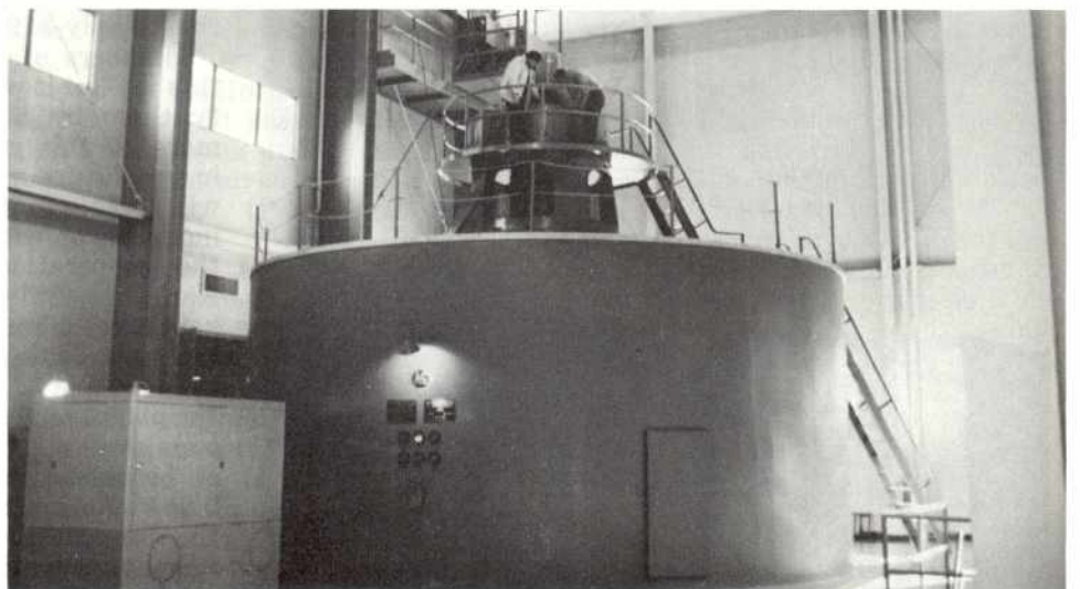
This is an "inside" view of the Donnells power house and generator.
