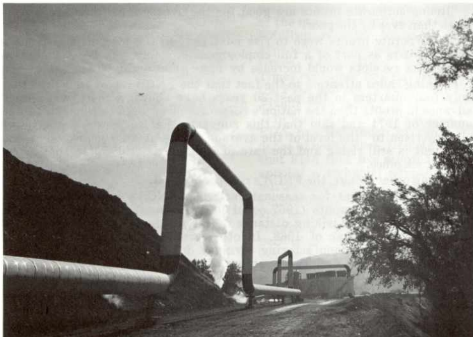
These expansion loops carry geothermal steam from wells drilled to a depth of more than a mile and a half to Pacific Gas and Electric Company's plant at The Geysers in Sonoma County, California. The plant is located about 90 miles north-east of San Francisco.
