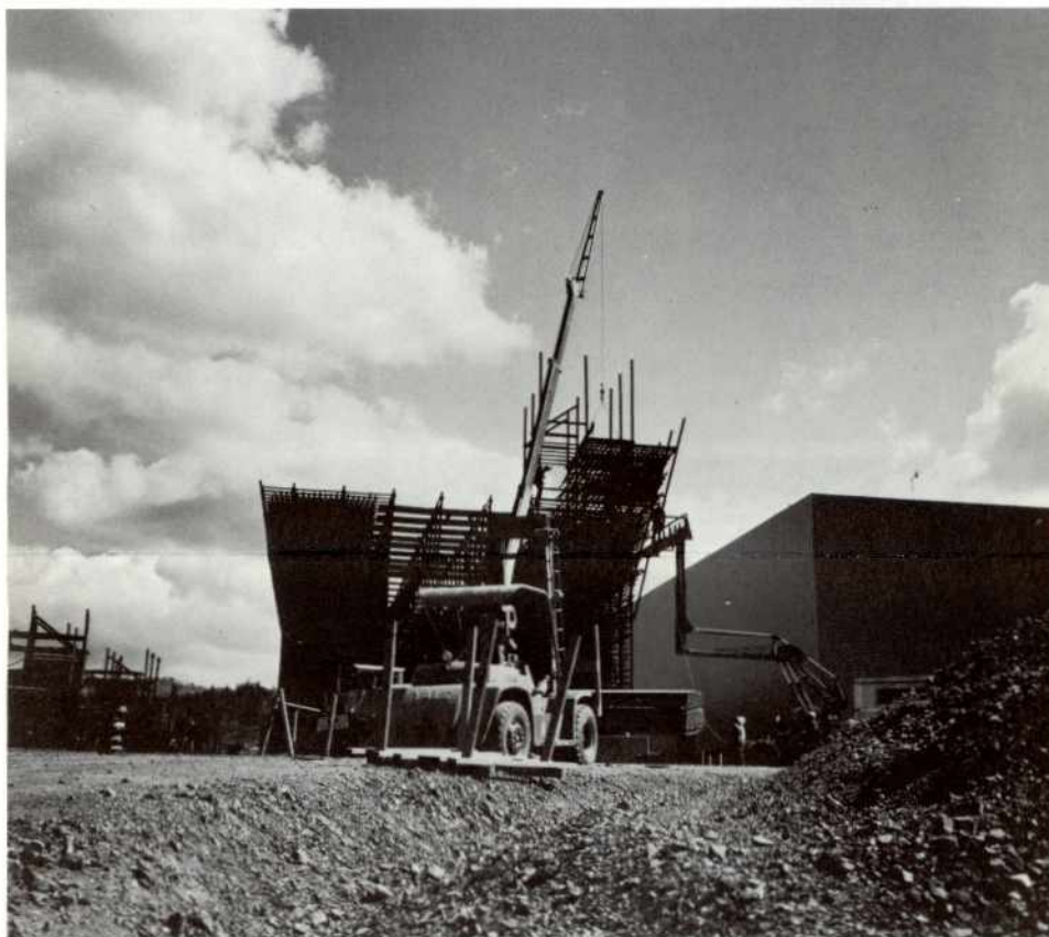
This cooling tower, when completed, will cool 29,000 gallons of water per minute from 118°F to 80°F with a 65° wet bulb ambient air. The fill, which you see being lowered into place, is made of polypropylene plastic.
