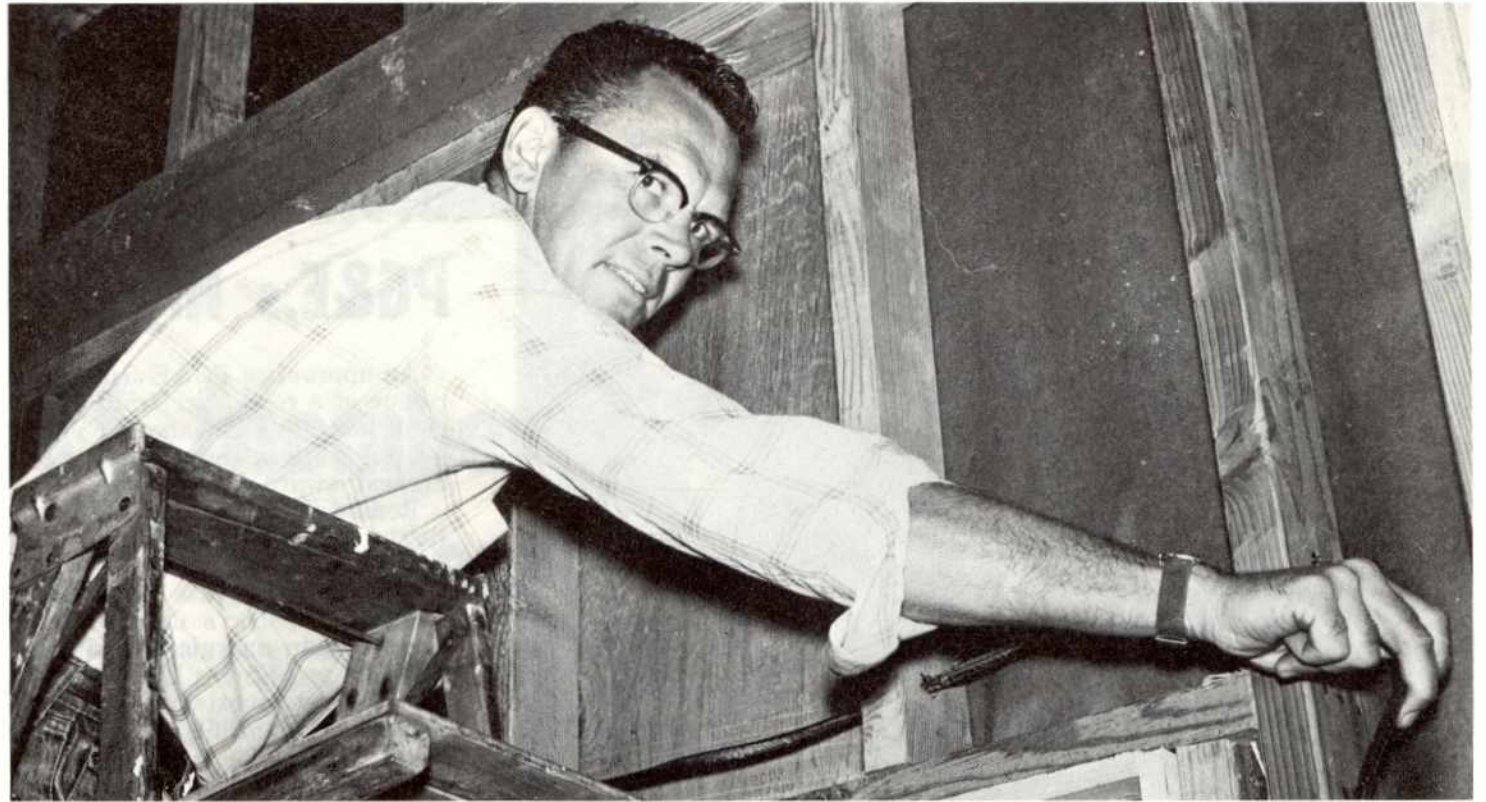
This picture shows us Bob Castle as he strings the wire in the new Teen Center building.
