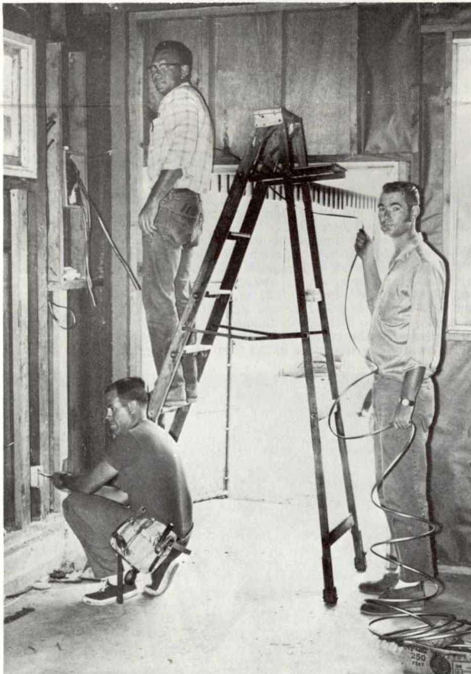
Shown above are three of our members working on the wiring project. Kneeling is Virgil Hood, Electrician and Shop Steward; on the ladder we find Bob Castle, Electrician and behind him Gary Barton, Electrician.
