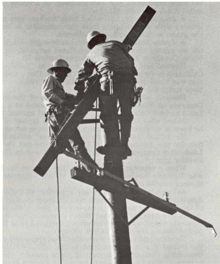
Two unidentified apprentices are shown working on a problem involving an Alley-arm at the McCloud-Pit Apprentice Lineman School.
