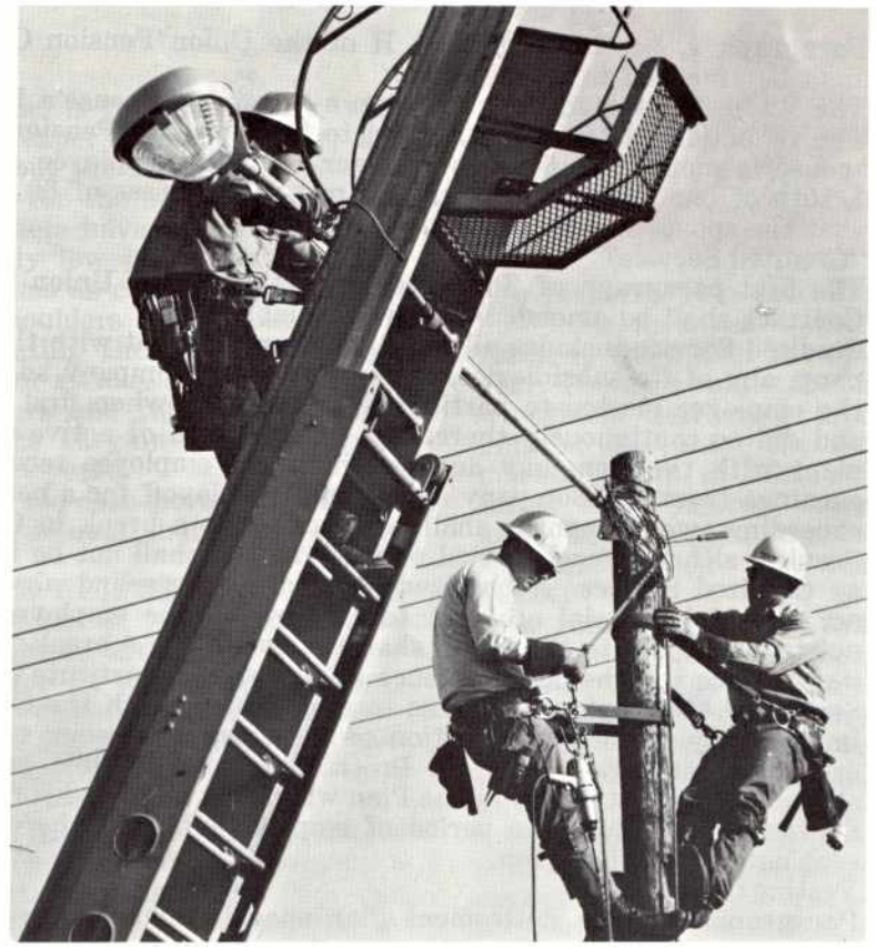
Left to right, Jim Kuhn, Sub Foreman, John Slater, Appr., and Al Kellar, Appr., are currently assigned to the San Leandro area replacing and installing street lights.
