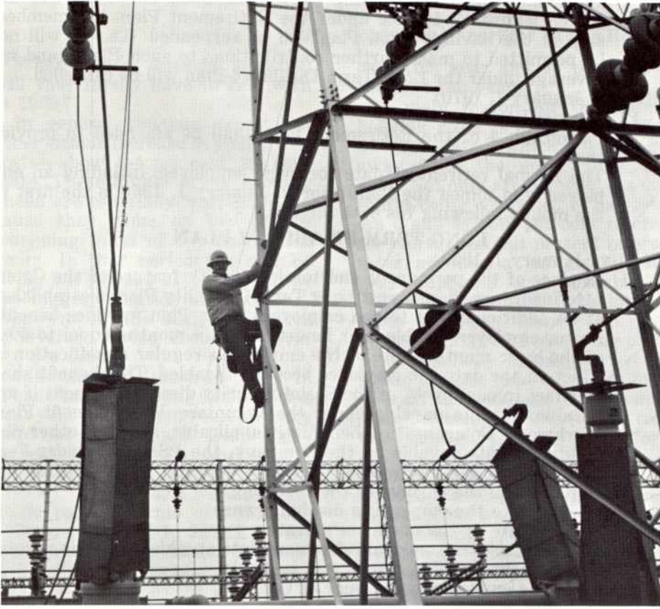
Monty Mitchell, Appr. Elect. at Newark Sub, is shown climbing a tower to begin work on insulator replacement.
