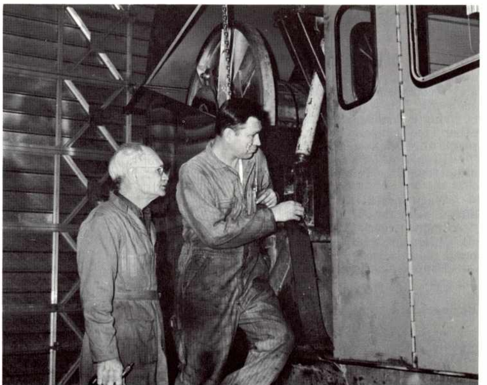
Del Hatfield, left, Davis Unit Chairman, is working with Guy Ross, Equipment Mechanic, on a special puller for heavy cable on underground work.
