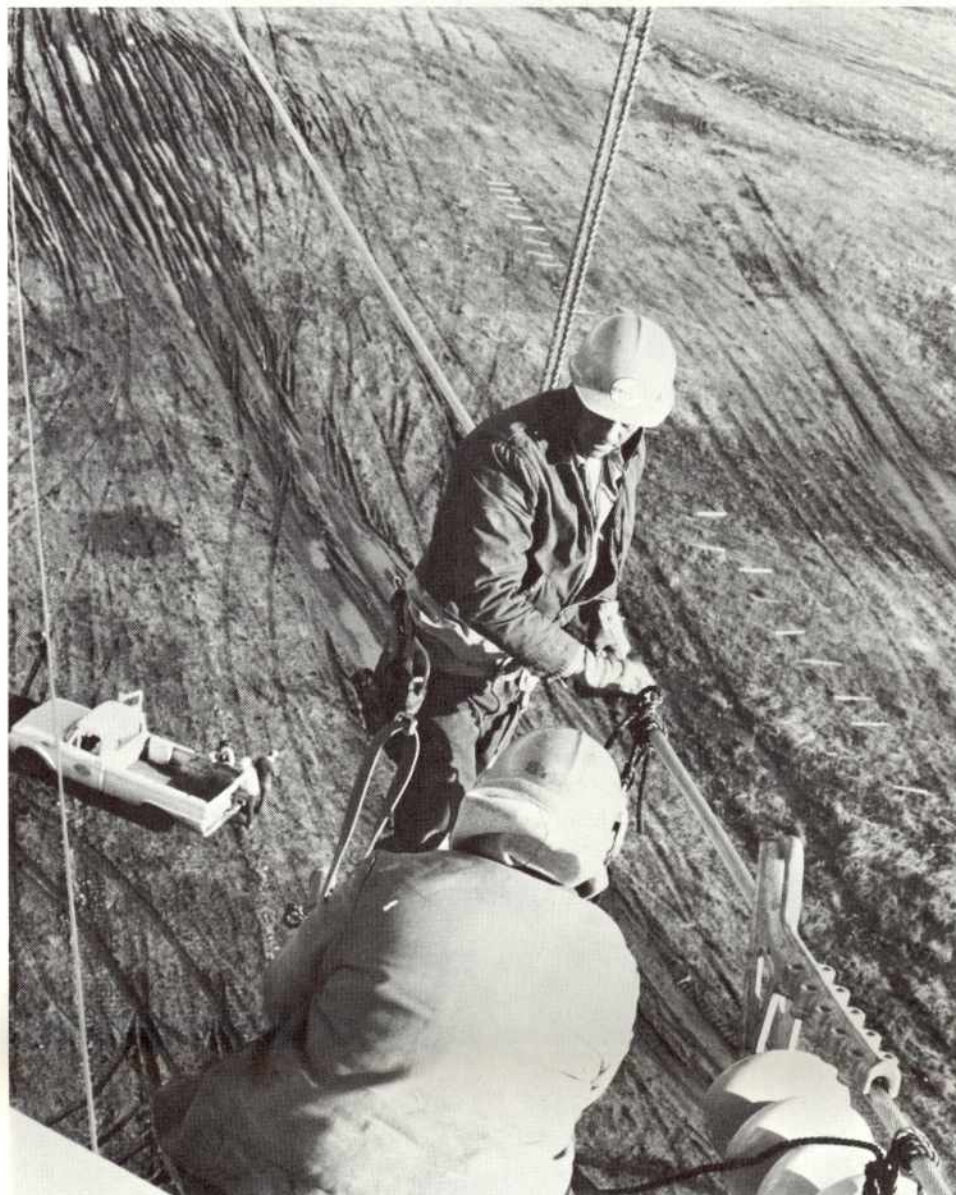
Outside Linemen George Shinn, top, and Bill Branson dead-end the 220 kv conductor on a tower of the Oroville-Thermalito-Round Mountain transmission line. "That's not a toy truck on the left," reports Business Representative Ron Reynolds who donned his Lineman's gear again to take this photo, "that's the real thing."
