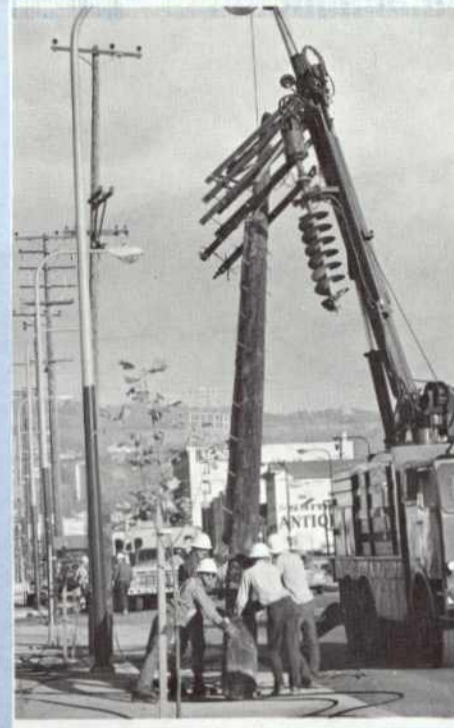
Down comes one of the 67 poles removed by PG&E crews during the conversion of Berkeley's University Avenue to underground.
