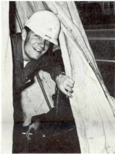
Tommy Norlen emerges from the tenting protecting the cable splicing operation at 4th and Wells in Reno.
