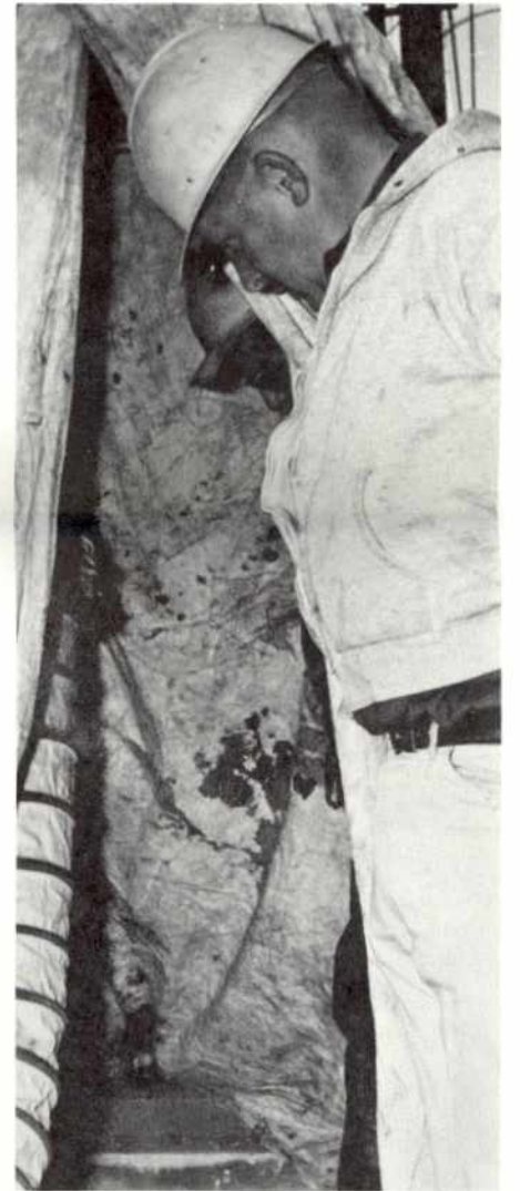
Harry Mewes looks down into the manhole to check on the progress of the cable splicing operation.
