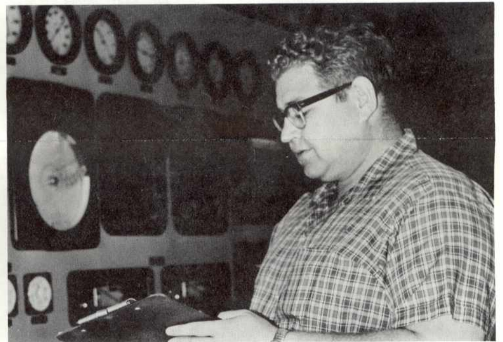
Emergency Relief Operator Lee Jones takes the hourly boiler readings from Unit 2's control panel.
