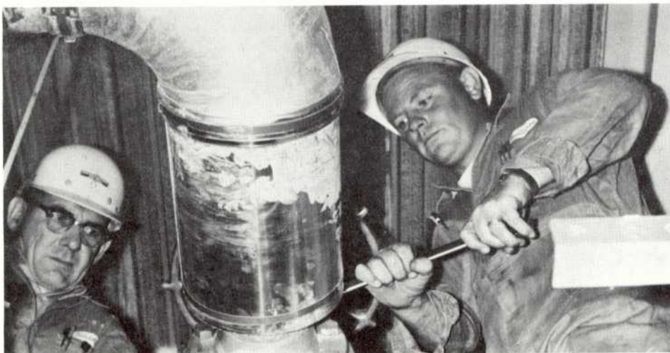
John Gondolfo, left and Al Dallimore tighten the flange on the check valve for the auxiliary boiler discharge.
