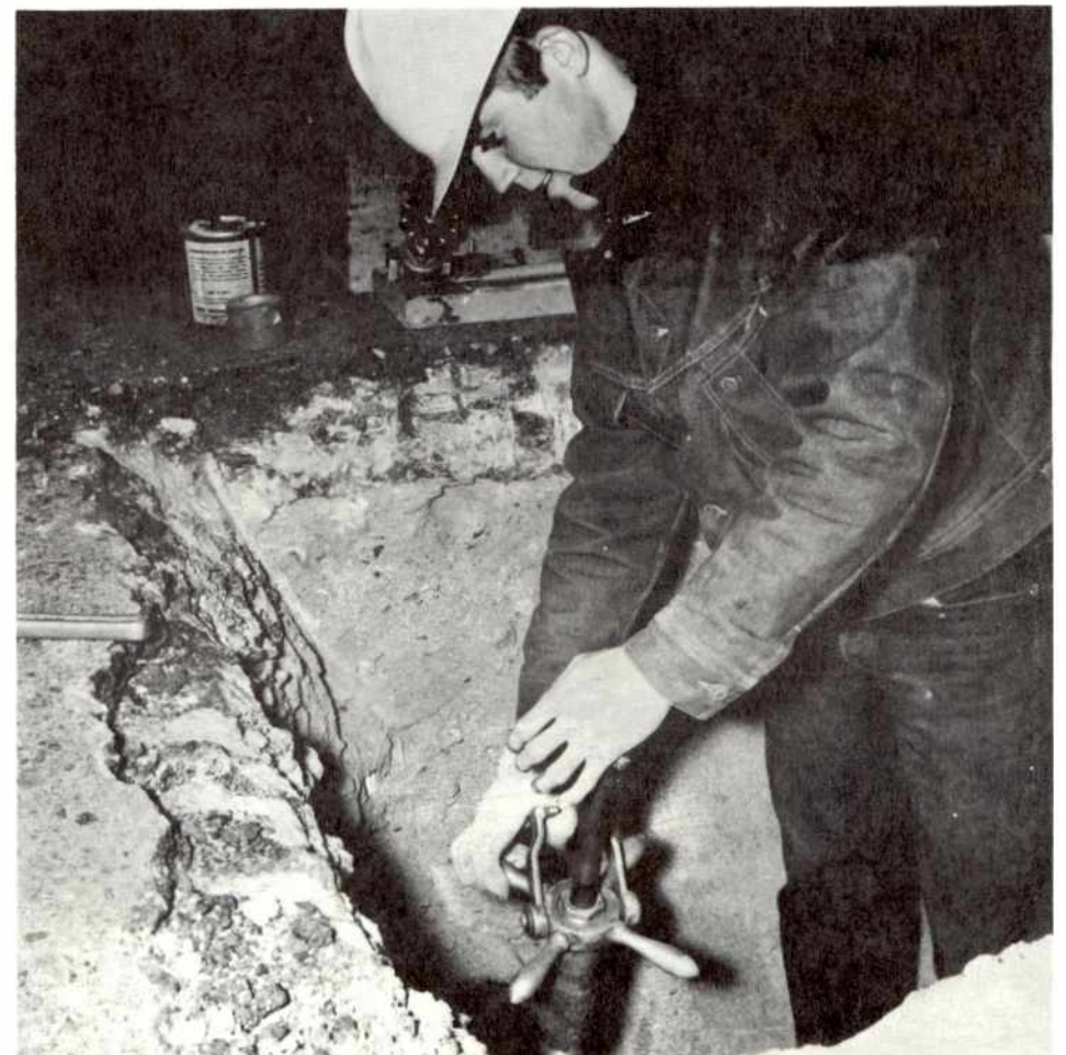
Ken Hawkins uses a Mueller tee to tap the 3/4 inch gas service into the 8 5/8 inch gas distribution main.
