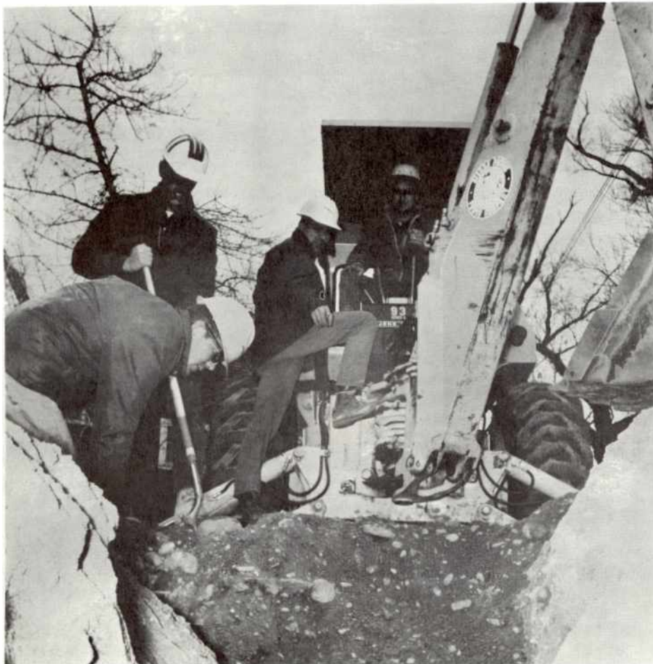
Walt Bettencourt points to where he wants backhoe operator Jack Larramendy to make his next pass as John Dupratt clears some of the sand away with his shovel. Other members on the crew not shown in this picture are Wimpy Rupp and Ken Hawkins.
