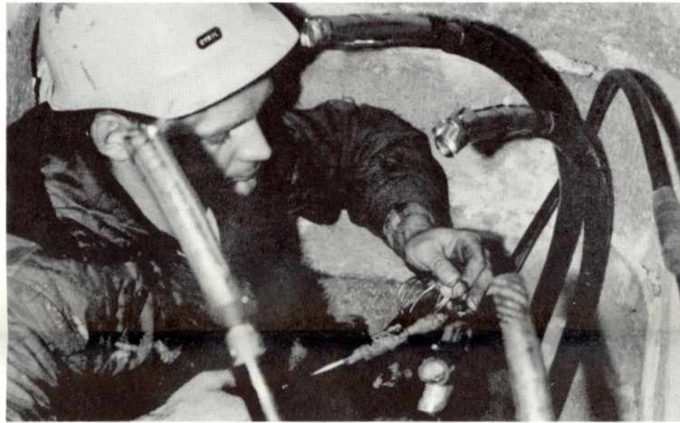
Cyril Escallier works on the 5 kv cable splice required by the undergrounding for Interstate 80 through Reno.
