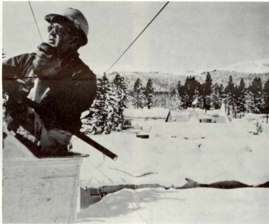
Shop Steward T. Bartl cuts a 14 kv jumper at South Shore, illustrating that if the Company does not serve all the way from the Sierras to the sea, it certainly serves from the sands to the snow.
