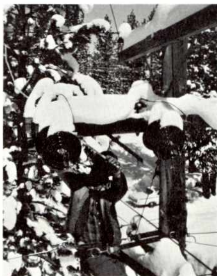
At Lake Tahoe, a 4 kv jumper is installed by Sierra Pacific Lineman Frank Anderson and the bucketman who took this picture. See page three for more pictures of The Sierra Pacific Story.
