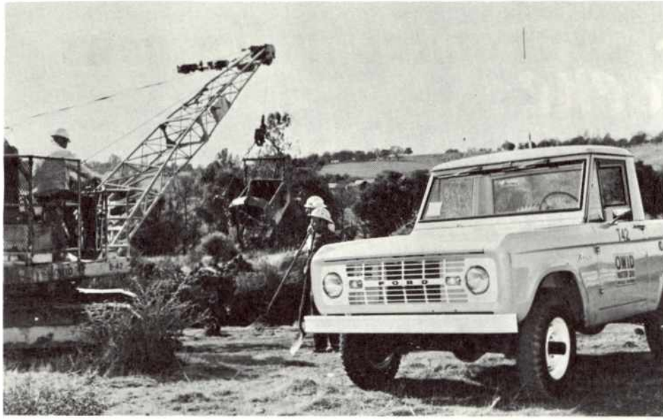
Ditch Tender Andy Proschold and Utility Plumber Ken Graves assist Equipment Operator Wayne Brewer on the dragline operation. The new retirement plan with its employer-paid past service benefit is a valuable provision to Andy who hopes to retire soon. OWID will match the employees' 3 per cent contribution for current service.
