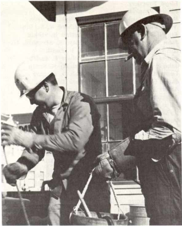
Senior Line Truck Driver George Koskela, right, and Apprentice Lineman Mike Perryman work on Scannell's crew at 22nd and Minnesota, near Potrero Hill.
