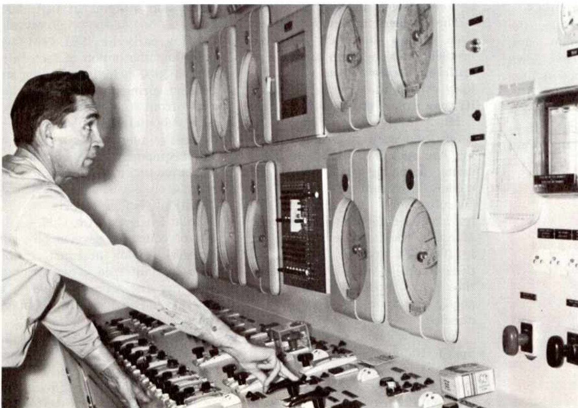
Senior Control Operator Bill Hamil "sees" the City's needs in the electric load it demands of the new Potrero Power Plant.
