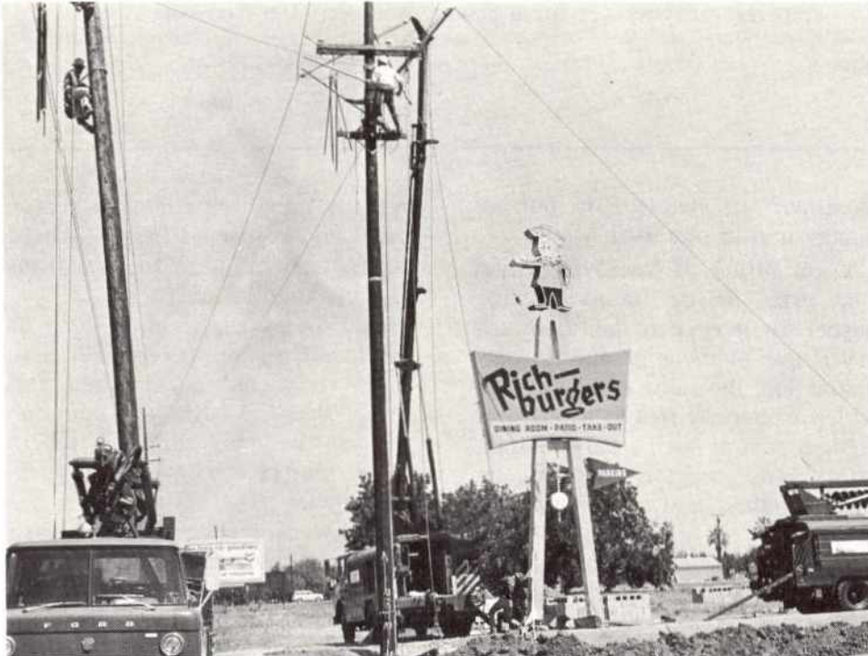
San Jose line crews transfer this 12 kv "hot" line on Winchester Road. Seen on the pole at left is Subforeman Robert Richards, and on the other pole, Lineman Bud Gaffney. Not seen in this shot, but working above these men on the two poles are Lineman Norm Shirle and Jim Hassett.
