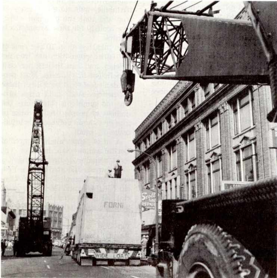
1. The prefabricated, concrete transformer vault arrives at 19th and Broadway, Oakland, accompanied by two 90-ton cranes.
