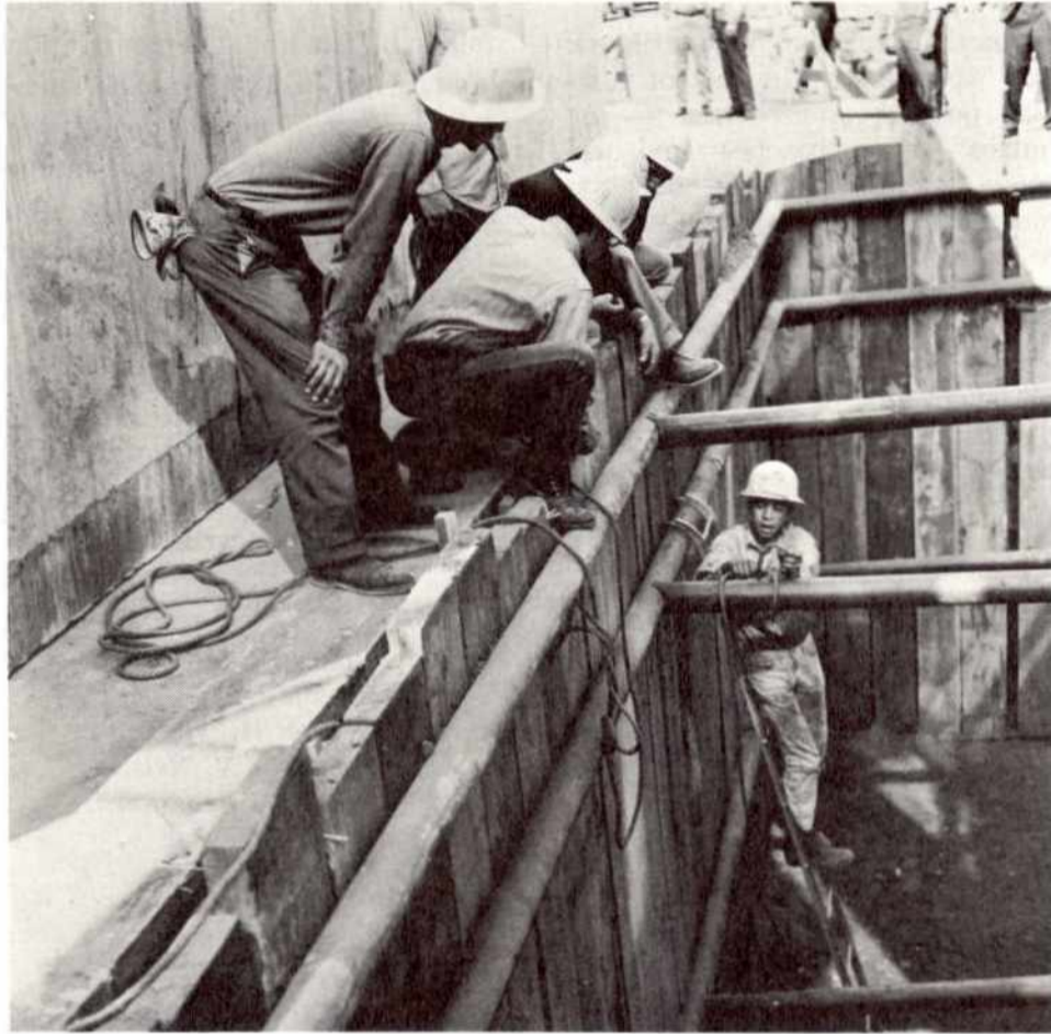
5. G.C. crew members rig lines to the steel cross braces before the twin cranes raise the vault, at left, and swing it into place.
