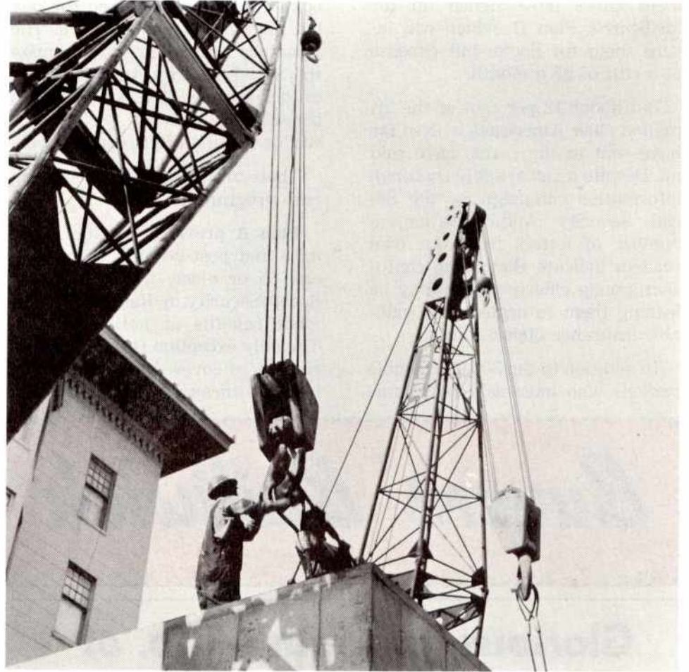
3. The chokers go on the hooks of the huge mobile cranes used by Bigge to swing the vault off the lowbed truck and into place underneath the sidewalk on 19th Street.
