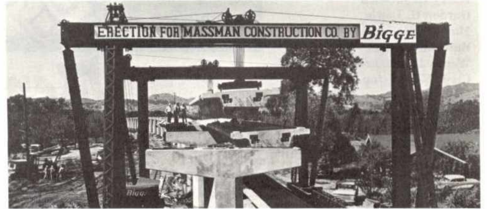
A gantry built specially for the Bay Area Rapid Transit project lifts a 100 ton precast concrete girder into place between two T columns. The girders, each 80 feet long, are being installed on a section of Diablo Test Track in Walnut Creek. This design will be used for the 31 miles of aerial structure in the 75-mile system.
