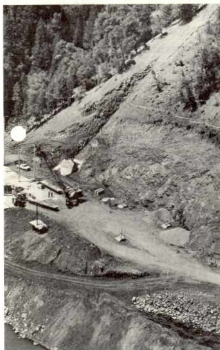
Cloud-Pit Powerhouse under construction for the switchyard which is being built by Local 1245 under the contract. Detail shows the pull-off location for the transformers.
