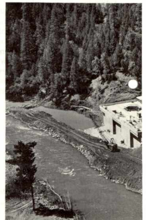
An aerial view of the construction and the site that will be built by men like the Joel Smith dispatched to the new line constructors' agreed structures erected above the
