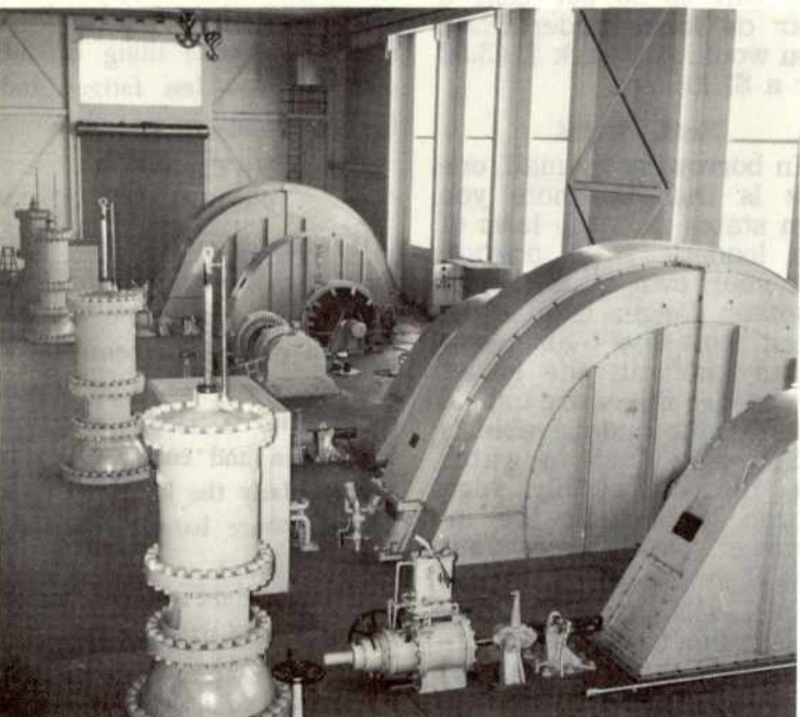
3. An inside view of the Electra Powerhouse taken from one of the top decks. Two of the three units are visible. Each has a generating capacity of 30,000 kw.
