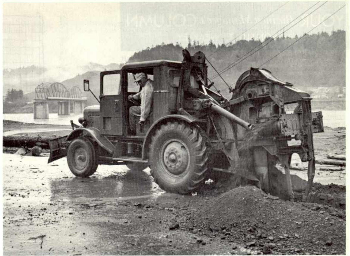
The force of the December floods in Northern California is shown by the wash-out of the South Rio Dell Bridge on the Redwood Highway in Humboldt County (background). In the foreground, Fitter Salvatore Mylie trenches through the pavement to restore gas service to residents of the flood-stricken Eel River area.
