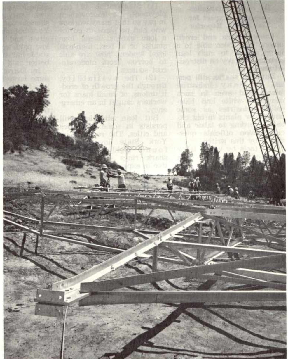
Northeast of Chico, G.C. crews build one of the 500 kv AC lines through difficult foothill country north to Shasta County.
