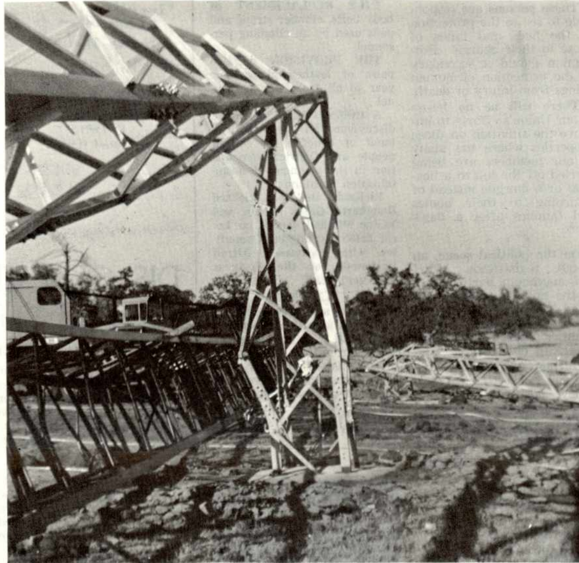
The mobile crane is framed by a twisted tower leg, top, and the crane's boom, bottom. The other tower leg is shown laid out from its footing at right.
