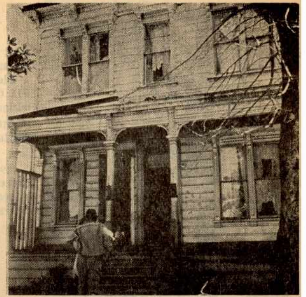
19 children live in this house. It is of a post-Pacific Heights era but obviously has not been kept up or inspected so well.
