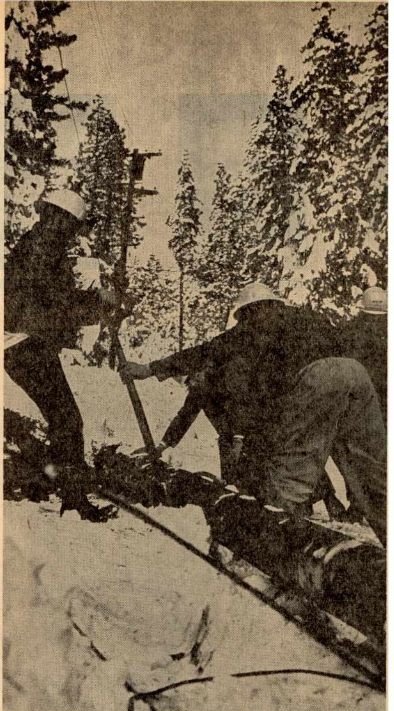
A fallen pole is manhandled by this crew in the Twain Harte area after the storm.
