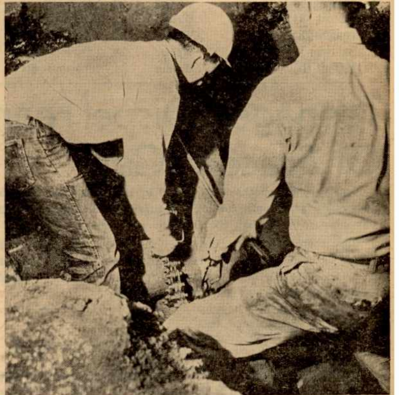
Fitter John Turner, left, and James Dietz use a hydraulic pipe cutter in order to remove a cast iron gas main and replace it with an 8 inch steel main. The location is in the outer Mission District of San Francisco.
