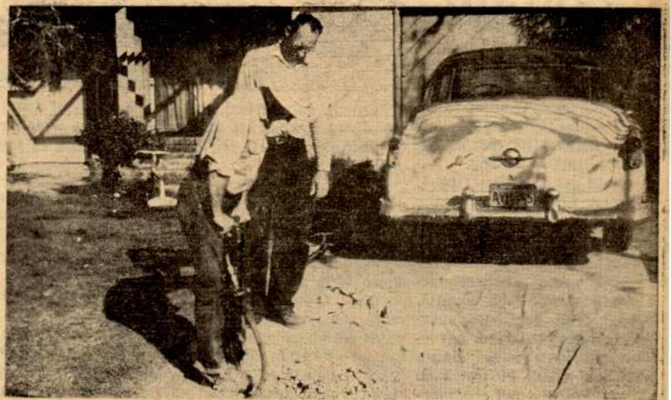
The "detective" work of the crew indicated that the leak was under this driveway so after informing the people in the house the pneumatic drill was brought out. (Car had dead battery and was not being used).
