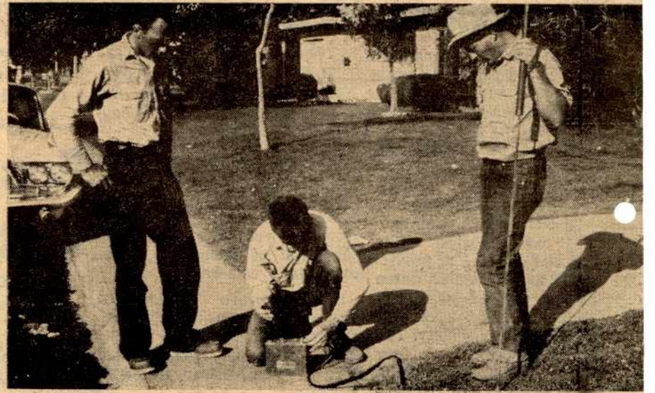
Here Seibel is using the "sniffer" to determine the location and heavier concentrations of the leaking gas. Bird is holding a probe—used to bore holes for the "sniffer."
