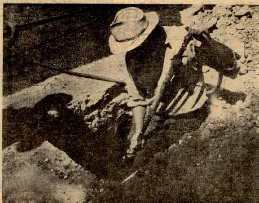
Refilling the hole requires that each layer of dirt be carefully tamped down to support the driveway properly. Bob Bird is operating the pneumatic tamper as the repair operation moves along.
