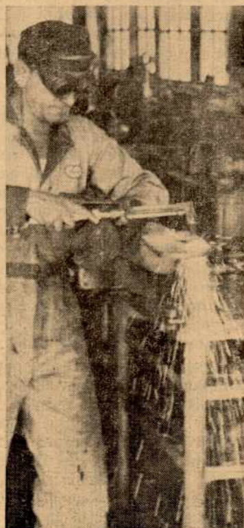
Rounding the end of a boom with a cutting torch is Samuel J. Brunner, Welder.
