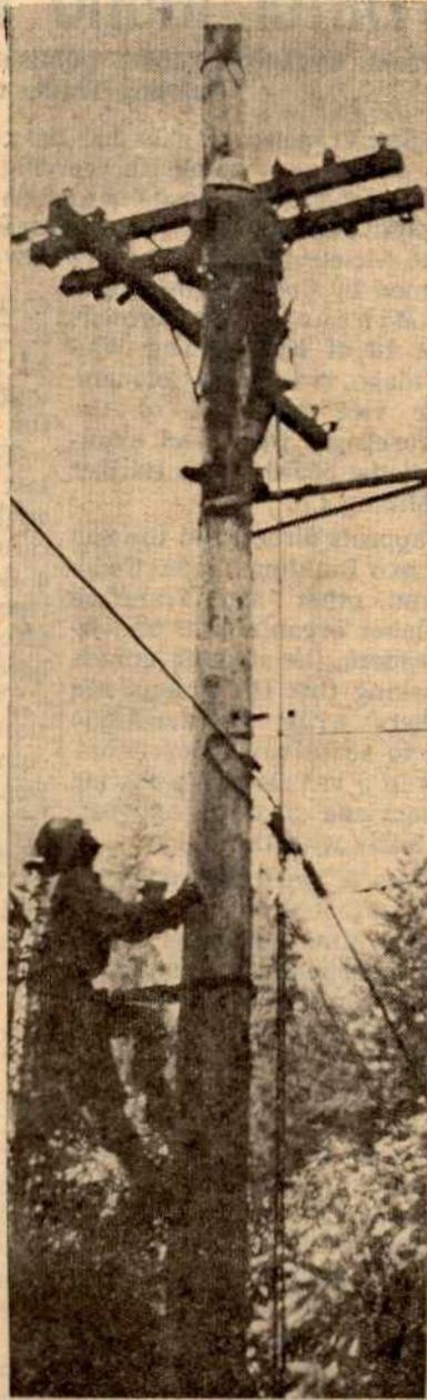
Line crew at Guerneville. Milt Hawes, Sub-Foreman, going up pole; Clarence Kelly, Lineman and Shop Steward, at top of pole.
