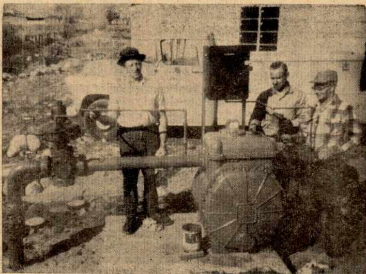
The "Grand-daddy" of gas meters on the Company's gas system, weighing over one-half ton, has a capacity of 10,000 cu. ft. per hour. Local 1245 members of the Service Crew shown are, left to right, Chas. Lercari, Bob Hedges and Sam Nagel.
