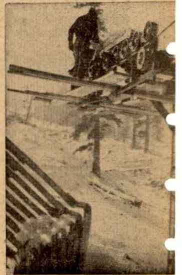
NEW SKI RIDE. Work on Valley ski lift which will cut valley floor, elevation 6,206-8,007 ft.
