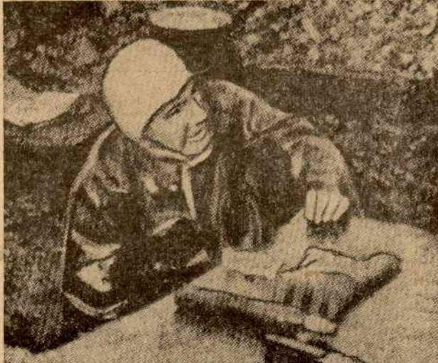
Although suffering from burns on his face, Local Union 1245 member George Lalla, employed by the Pacific Gas and Electric Company as a Fitter, re-entered an opening in a Berkeley street to shut off a gas main that had exploded into flame while he was repairing it. The accident occurred Dec. 15. (Exam. photo.)
