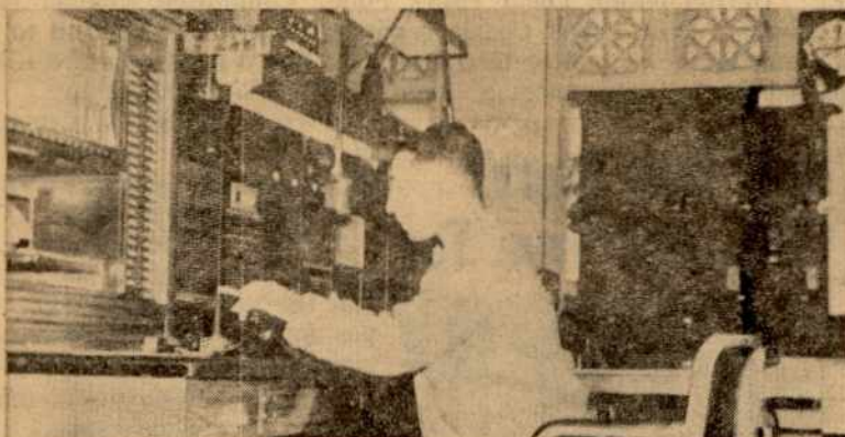
Ed Lomba at the PBX Board, where he assumes responsibility for Oakland's 1300 fire alarm boxes, among several other alarm systems, while on his 8-hour shift.
