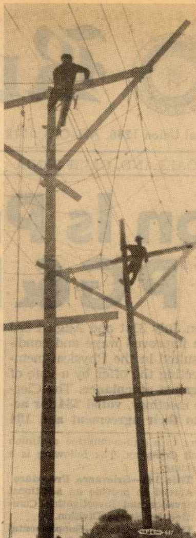
Here are Paul Troglia and Clyde Van Meter silhouetted against the afternoon sky on the Eastshore Freeway towerline heading into Station "J", Oakland. They are working on guard poles. Note protective nets. Crew headquarters are at Station "O" in Hayward.
