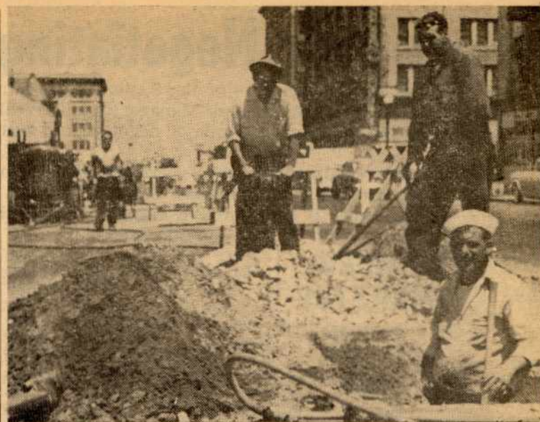
STREET SCENE, OAKLAND—General Construction gas crew is shown in this candid picture repairing a gas leak at 14th and Jefferson, Oakland. Let's have more of these on-the-job pictures for the "Utility Reporter!"
