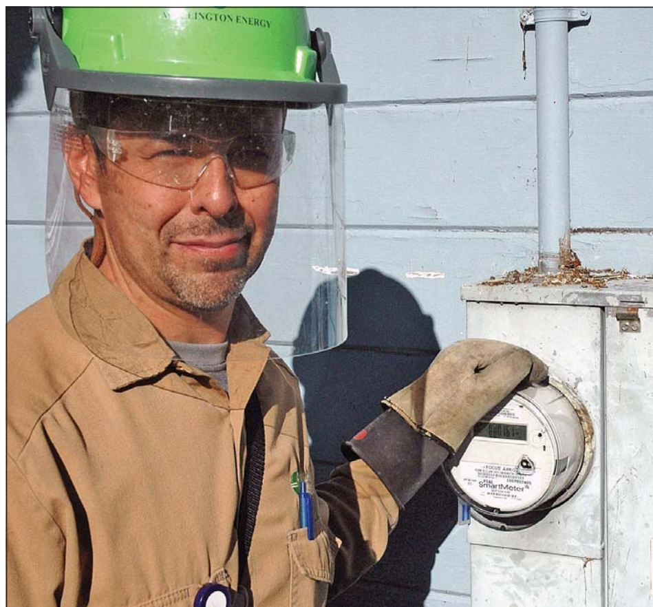
Wellington Meter Technician Orlando Miramontes removed an old PG&E electric meter and shows off the new SmartMeter he's installed in its place.
