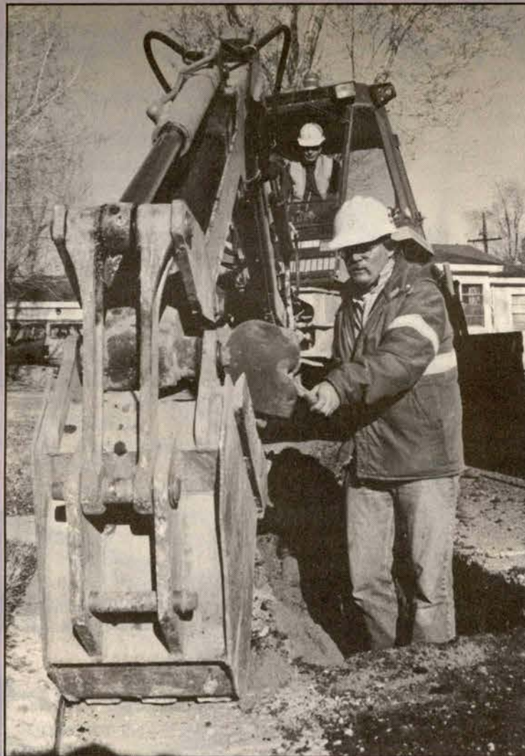
Jay Atwood, backhoe operator, and Alan Helm, heavy truck driver. (Photos: Eric Wolfe)
