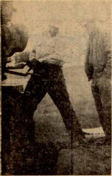
Hole-digger operator Al Dohs is shown digging a hole for a dead-man just outside the Divide Sub Station in the southern end of Coast Valleys Division, while Foreman D. J. Gosnell (at right) checks the operation.
